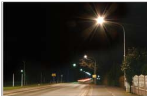
The modernized equipment, viewed from the opposite direction, with modern Koffer-line luminaires fitted with CosmoPolis 60W.
